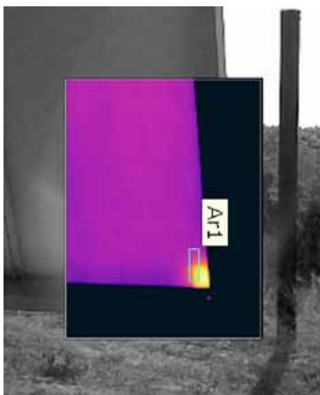
This Picture in Picture image shows a hot cell due to a shadow from the nearby alarm system.
