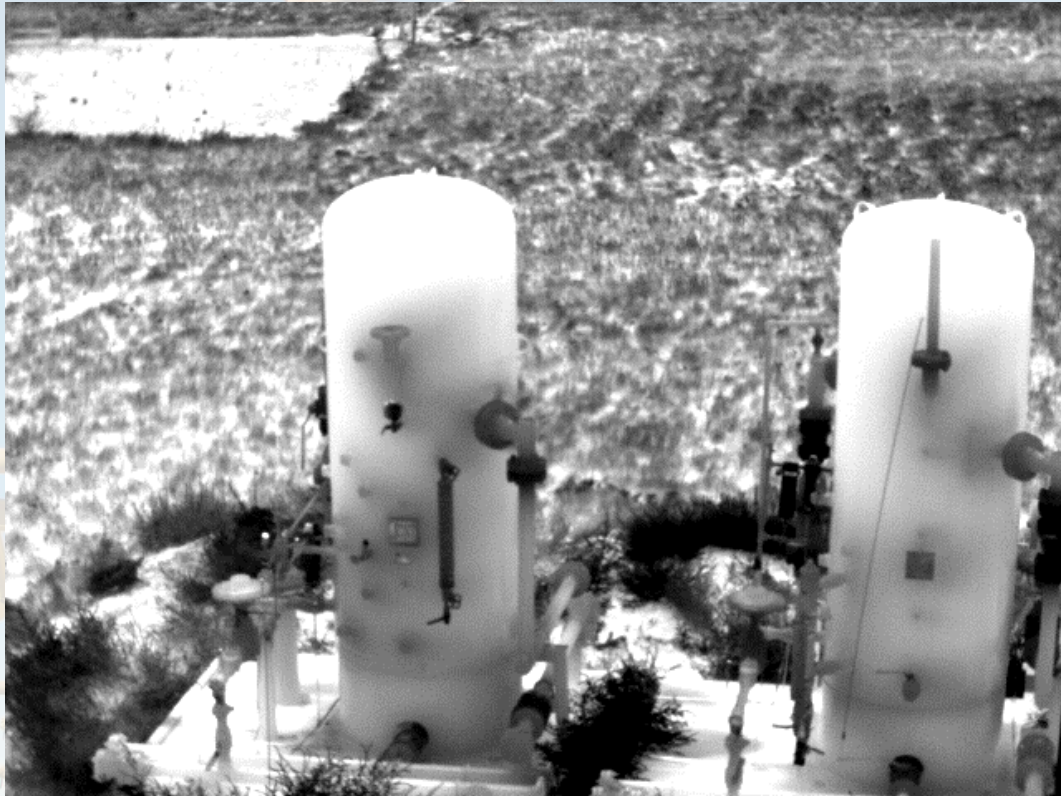
Separator LEAK at Flange
